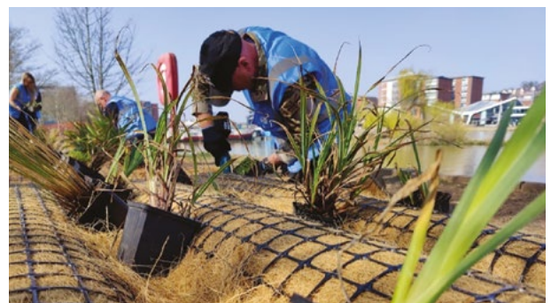
Lincolnshire Rivers Trust project to install floating biohavens in Brayford Pool in Lincoln city centre. Credit David Martin
